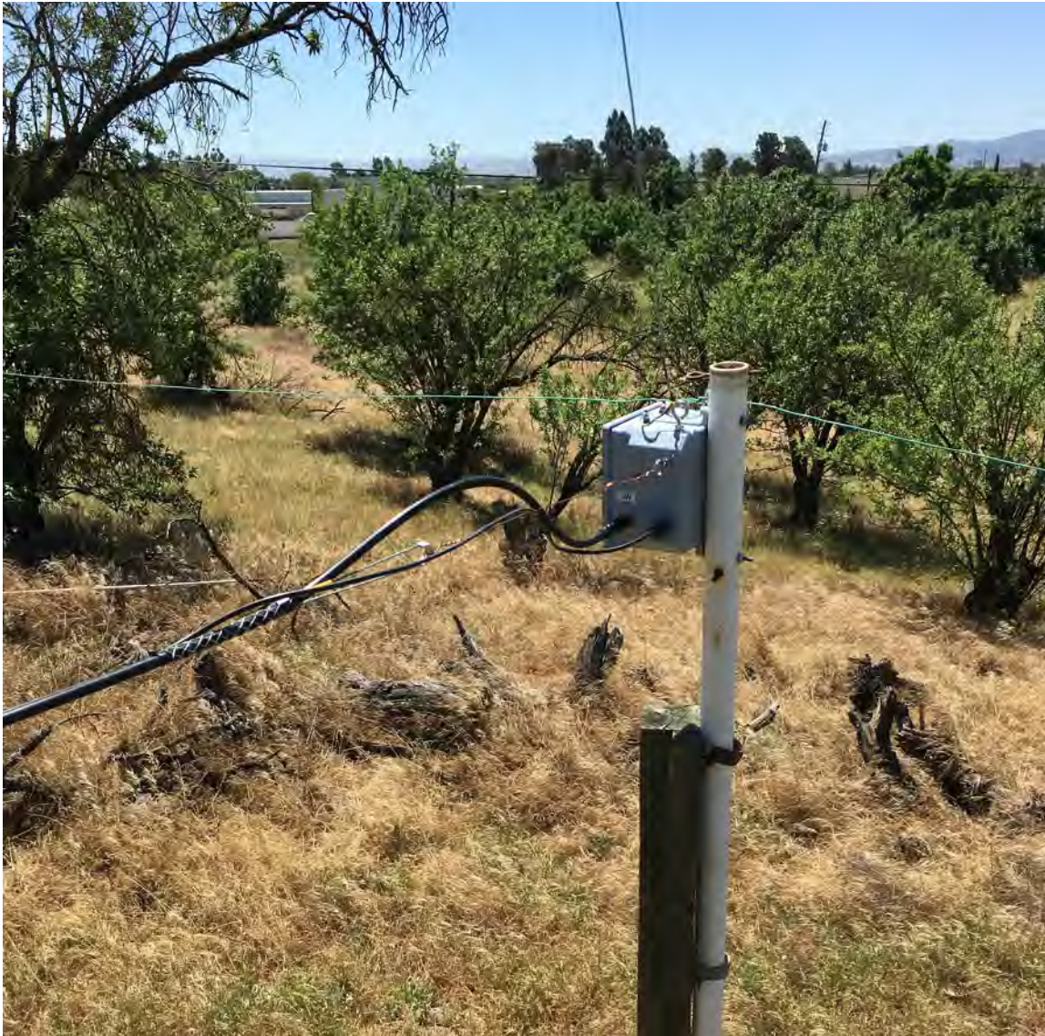
Figure 4. Antenna box installed. Feedlines have nice strain reliefs. This should hold up well. If only the wires would survive all that flexing the wind.
