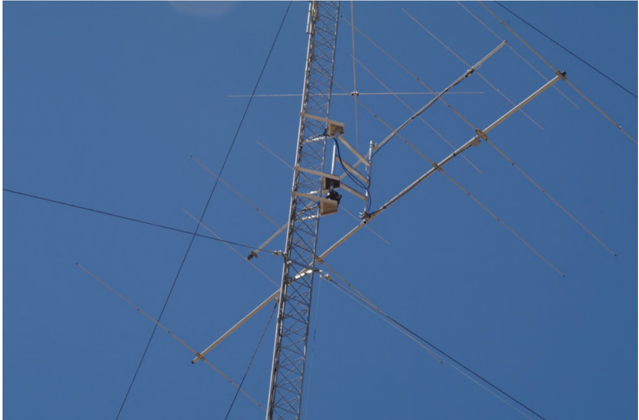
Figure 6. A swing-arm mount supporting two antennas. This one is fabricated from aluminum by Robin, K4IDC.
