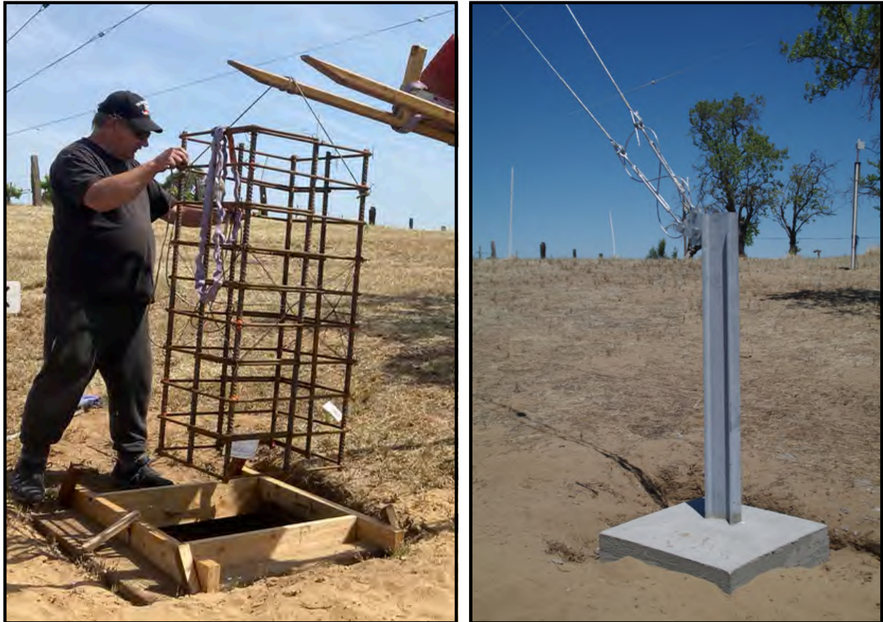
Figure 5. New guy anchors have a substantial rebar cage in the base and use galvanized I-beams that are designed to handle the full load with a large safety factor.
